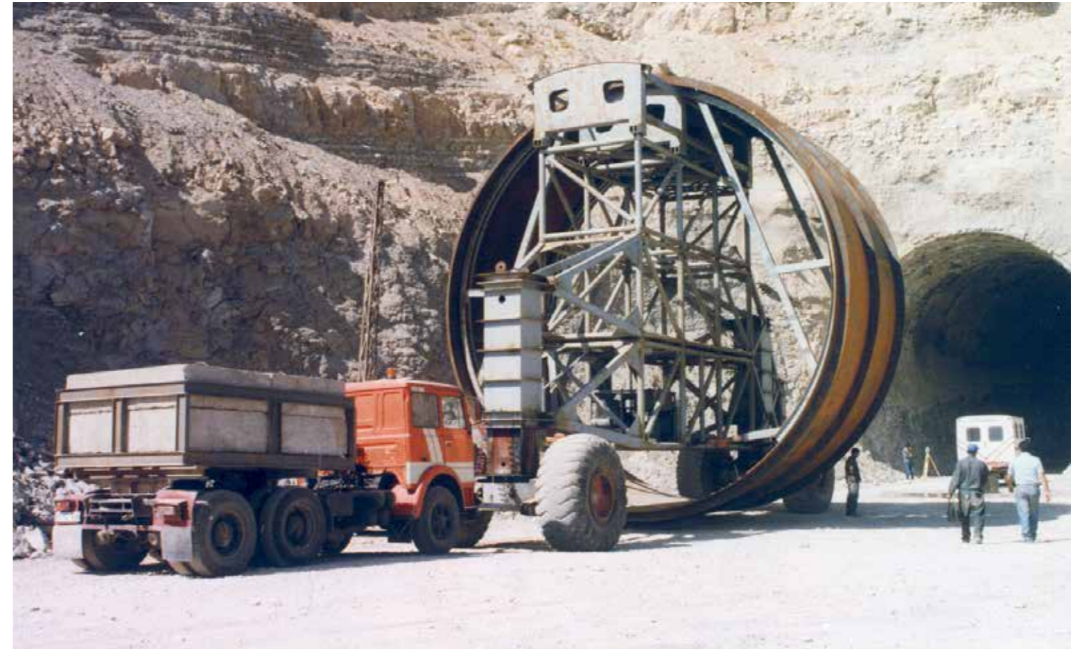
Batman DAM, Türkiye (3 x 63 MW) Diameter: 9.5 Mt.
