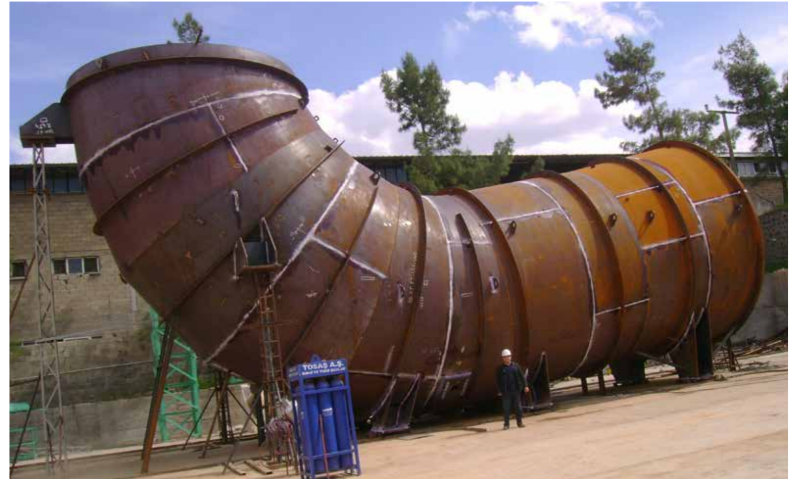
Yedigöze HEPP, Türkiye (2 x 158.5MW) Contractor: ALSTOM Hydro
