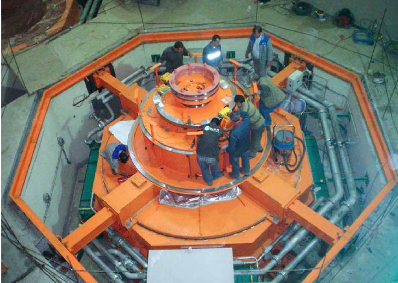
Darica HEPP, Turkiye (2 x 50 MW) Contractor: VOITH Hydro
