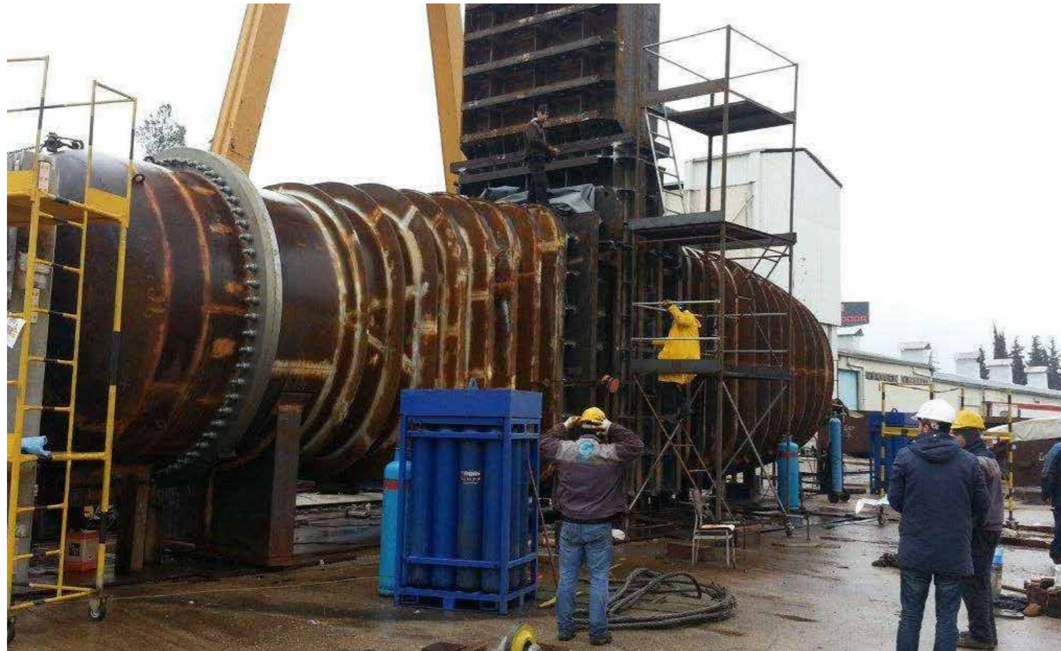
Artvin HEPP, Turkiye (2 x 166 MW) Contractor: ALSTOM Hydro
